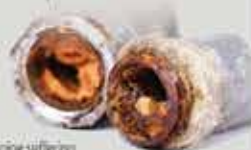
Example of pipe suffering contamination build up
